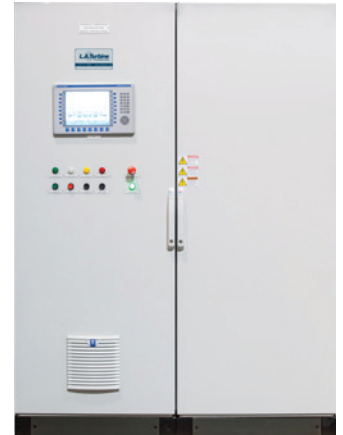
Remote Control Cabinet
